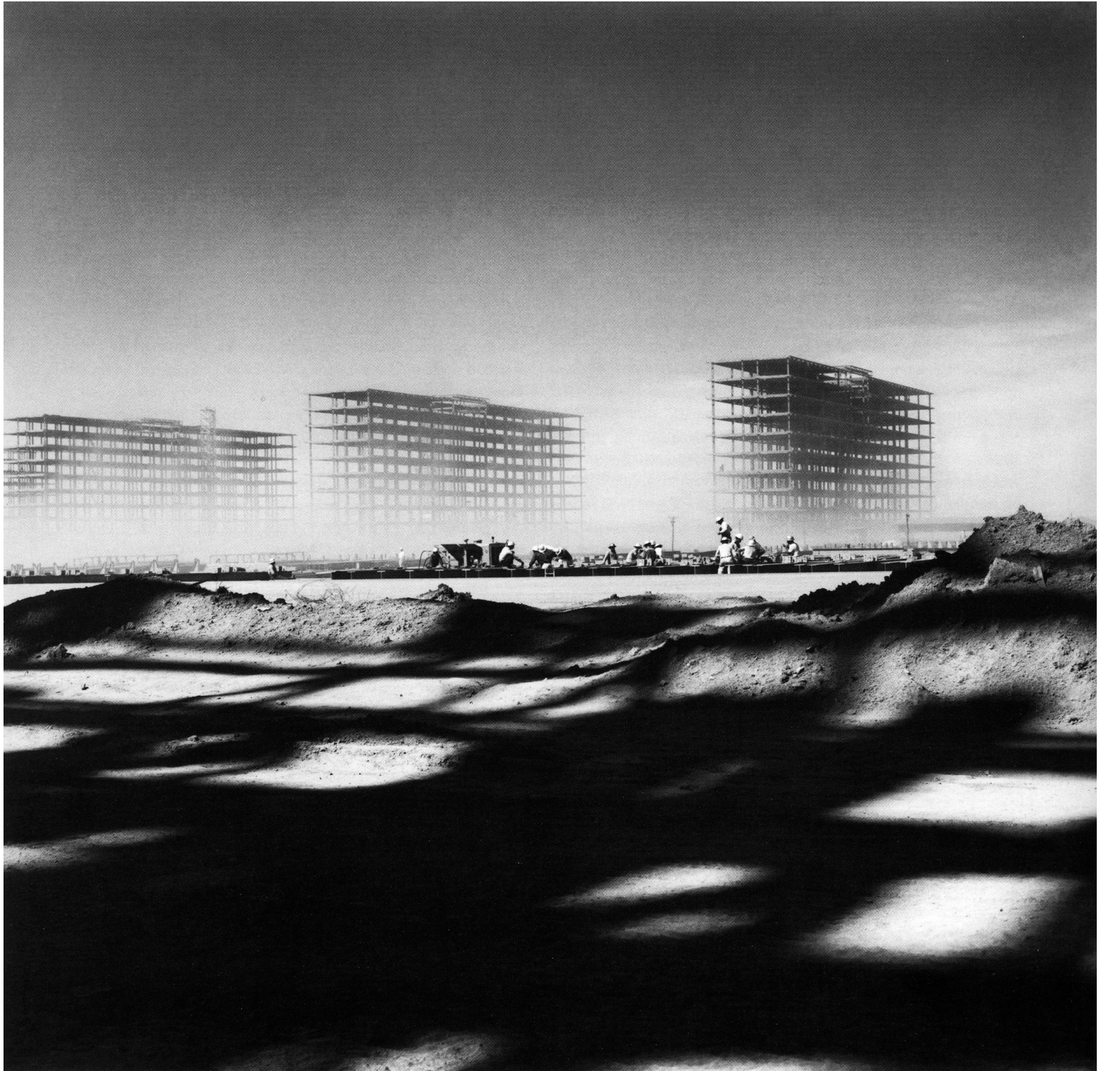
Figure 1. Marcel Gautherot, Steel-frame ministry slabs under construction, Brasília, 1958. © Marcel Gautherot, Instituto Moreira Salles, Rio de Janeiro.
